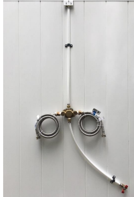
Back of Unit – Positive Balancing Valve & Hose
